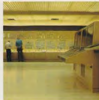
The central control room for the DataFreeway™ network is the access point for all of the data flowing in from every mill operation.
